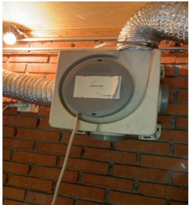
Ventilator TR achter
